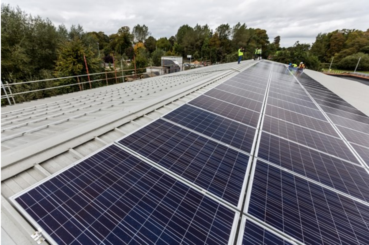
Figure 4: Solar Photovoltaic installation at Tipperary County Council building
