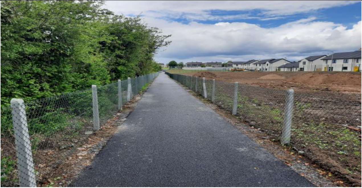
360m of existing walk between Mill Road and College Green housing estate, Thurles upgraded
