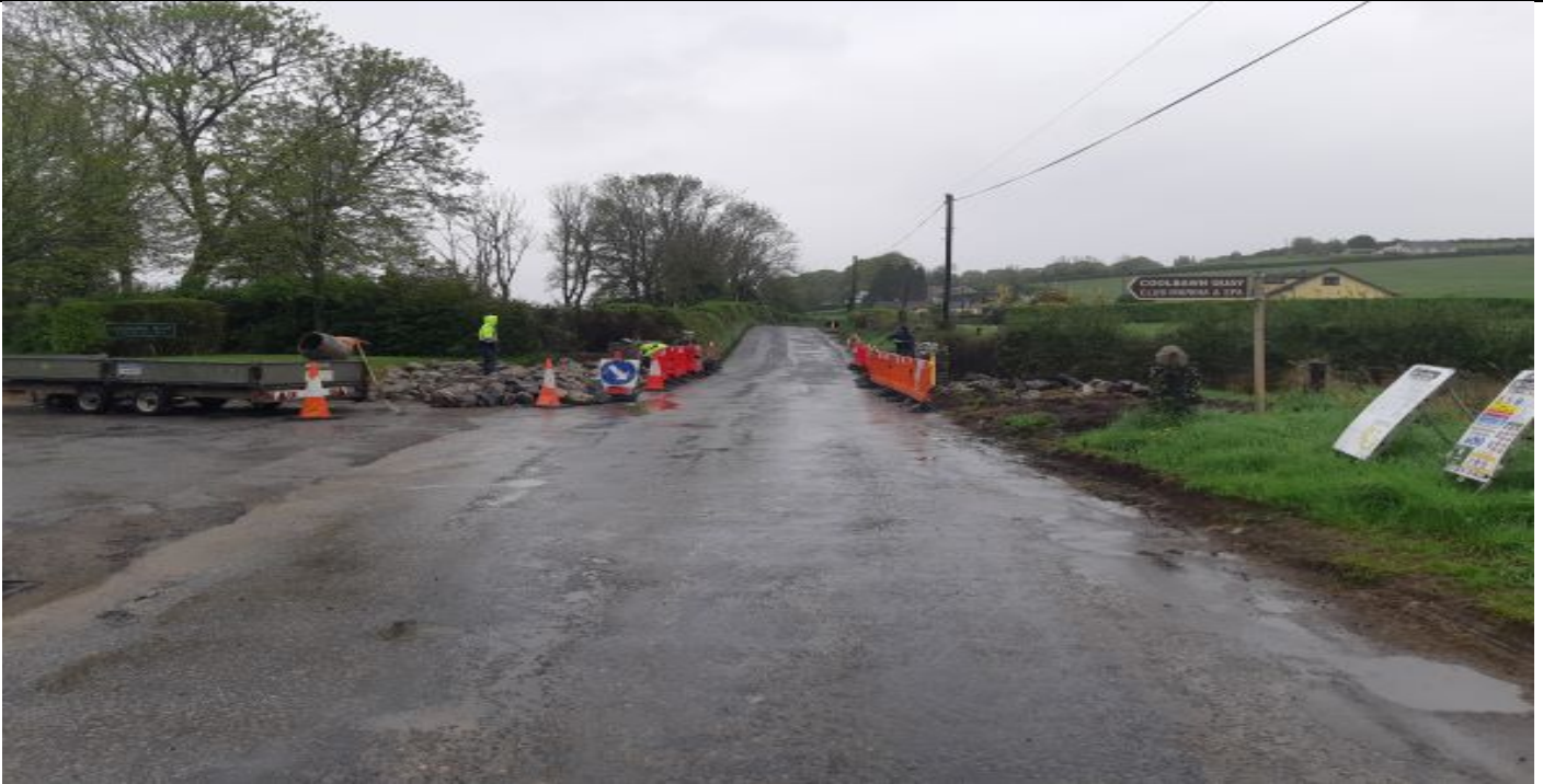
Rebuilding damaged parapet walls of a culvert under the R493 at Coolbaun, Nenagh, resurfacing to follow
